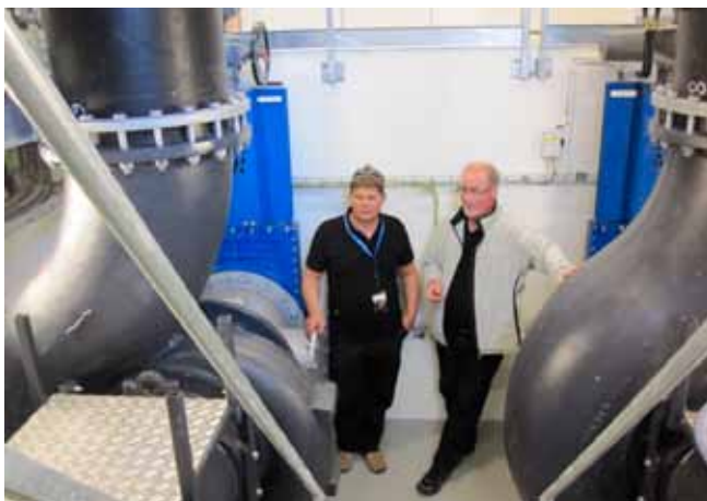
Project manager at Grundfos Pumper, Geir Nilsen and AVK project manager, Edgar Larsen in front of two dry installed Grundfos pumps each weighing 3,000 kg with a capacity of 780 litres/second. Also, two 400 kg immersion pumps have been installed – each with a capacity of 150 litres/second.
