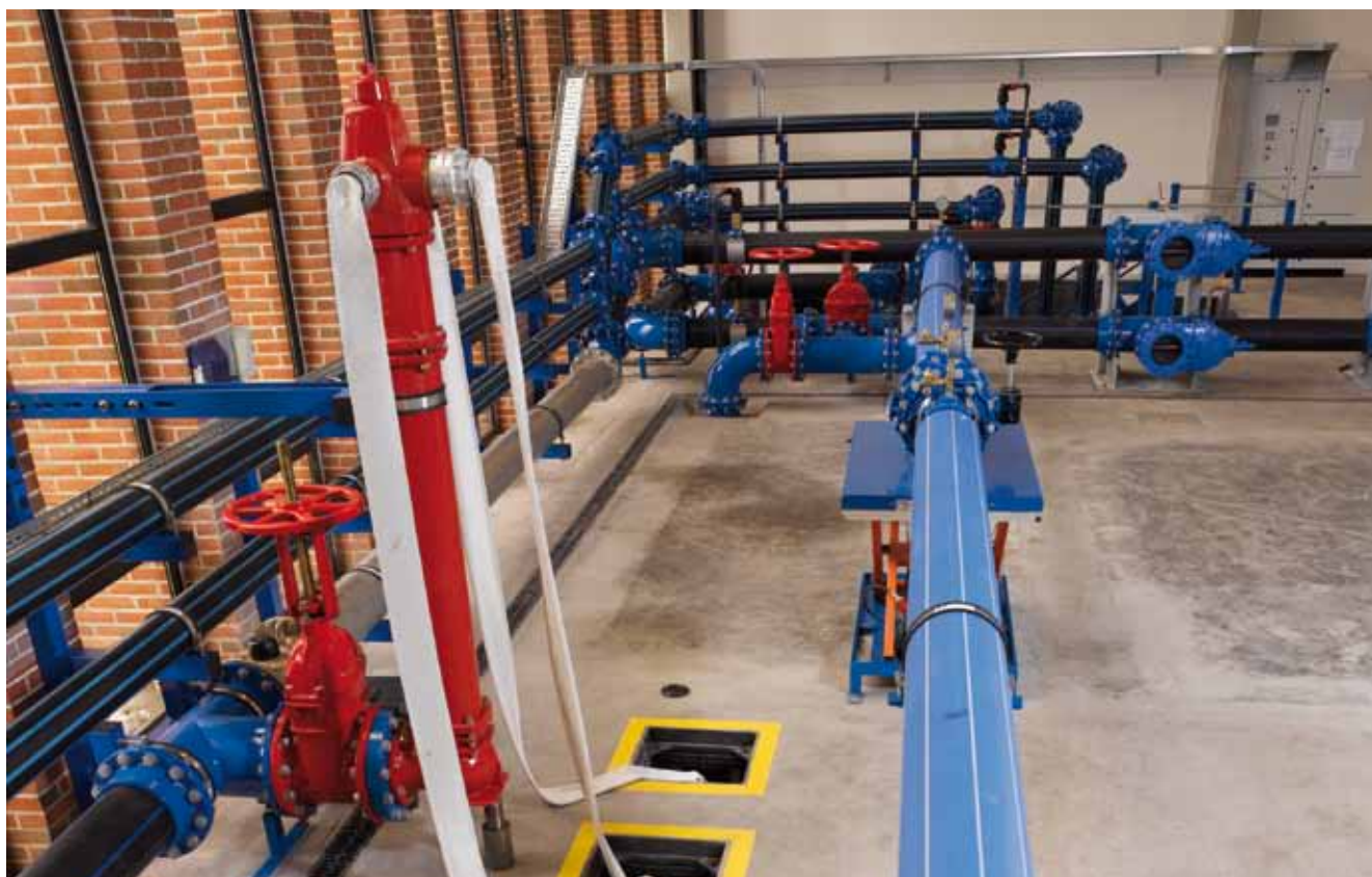
Hydrant test station. Here, the hydrants can be performance tested through one, two or three outlets. Most standards require specification of minimum performance, but here, we are also able to find the maximum performance.
