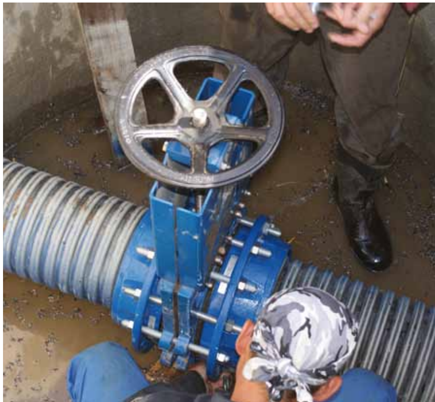
Installation of a knife gate valve and combi flanges in Russia. Sent in by Marina Kovaleva, Santeh-Servis.
