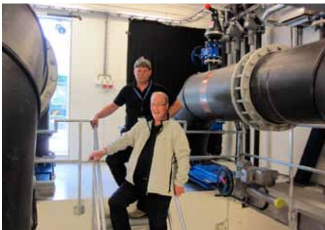
PE-pipes Ø630 have been installed in the pumping station. Here, in combination with knife gate valves series 702 and air valves series 701.
