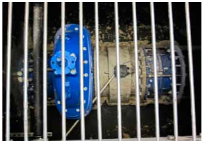
Fortunately for our valves, they have no idea of what await them when they leave our clean and cosy warehouses. This valve is attached with a water gauge and placed behind a grate. In addition, the valve is partly flooded by sewage water. We hope it will be much better off in its next life.....
