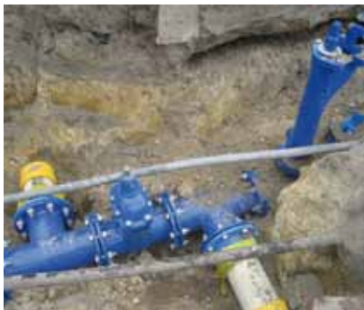
AVK valves being installed at the industrial area of World Valve in The Netherlands. Sent in by Peter Heijink, World-Valve B.V.
