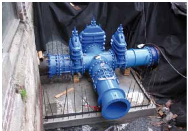
In the street outside the pumping station, the old DN600 cast iron pipeline has been connected in a newly built well. The well is 20 m 2 . Walls and roof were casted after installation of these three DN 600 gate valves series 06/30.
