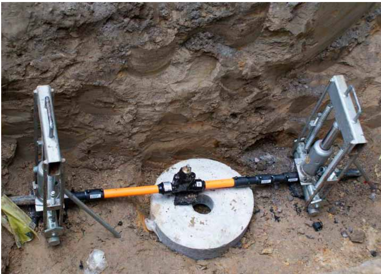
Installation of gas valves in Russia. Sent in by Volyntsev Maxim Vladimirovich, Santeh-Servis.
