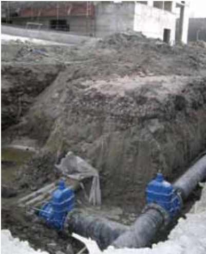
Installation of gate valves and dismantling joints in Russia. Sent in by Marina Kovaleva, Santeh-Servis.
