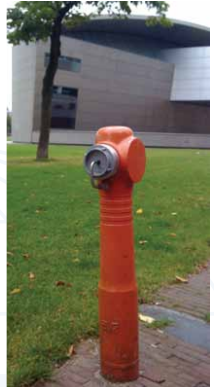
Series 09/90 fire hydrant - outside the Van Gogh Museum in Amsterdam, The Netherlands - sent in by Paul Hubbert, AVK UK Limited.
