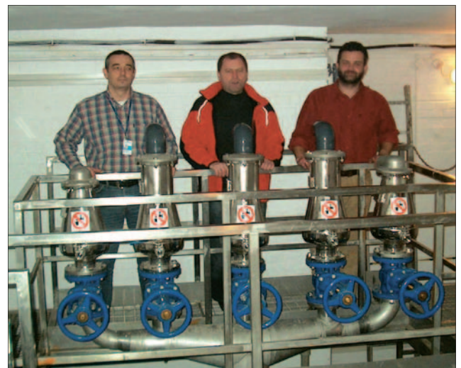
The two inspectors from Aquanet with Mirosław Kopyta in the middle standing behind the ARI air valves.
