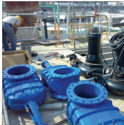
Hong Kong Shak Wu Hiu Sewage pump station
