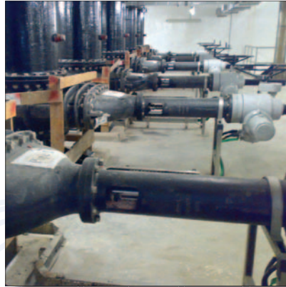
Hong Kong, North Point pump station
