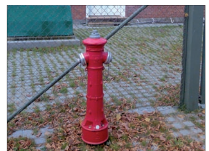
Nostalgic hydrant installed in Denmark. Sent in by Jens Jørgen Udby Nielsen, AVK International A/S.
