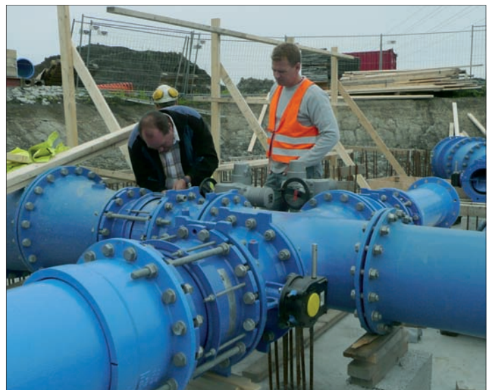
A Photo from Norway taken by Mr Per Ole Bakken, AVK Norge AS.
