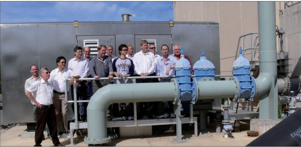
Port Adelaide sewage pump station
