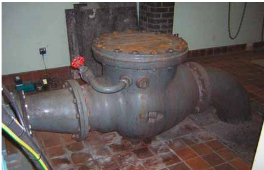
The original 1960's Glenfield Valves
