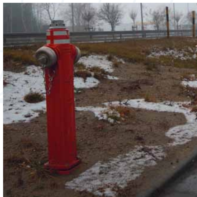
Installation of af series 84 fire hydrant. Sent in by Inga Wisniewska, AVK Armadan Sp. z o. o.
