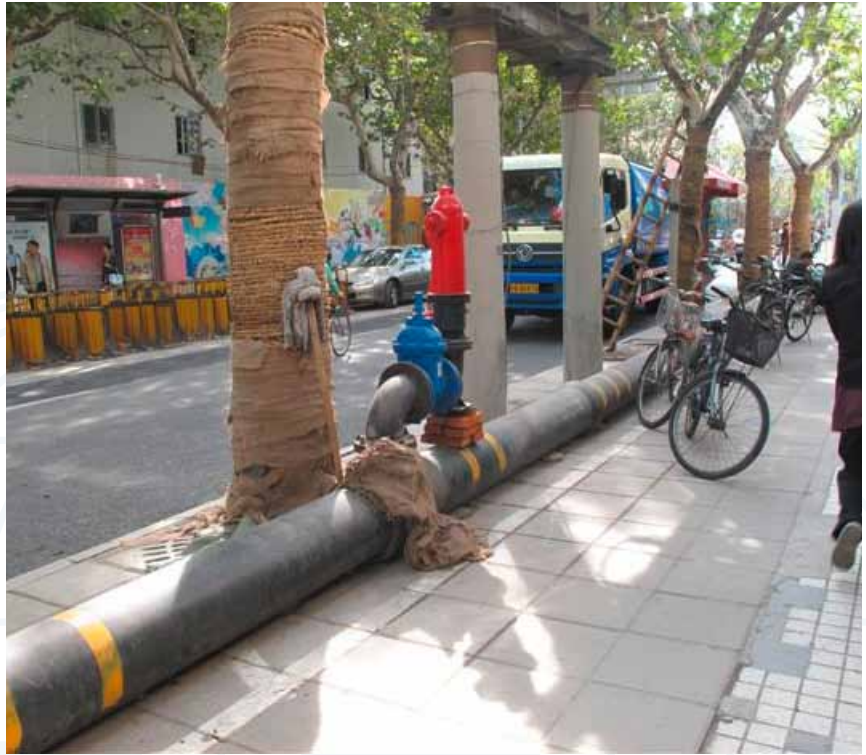
This AVK valve was installed on a temporary pipeline in the French area in Shanghai while the water distribution system was being renovated. Sent in by Jørgen Frederiksen, Teamprojekt, Denmark
