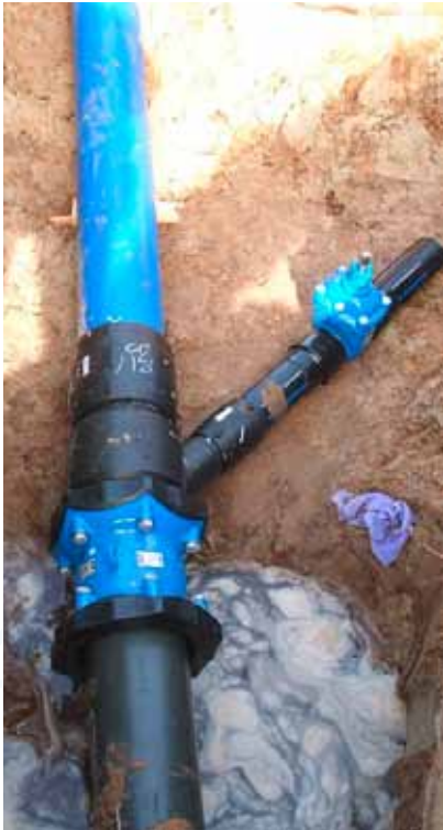
SupaMaxi™ installation. Sent in by Heike Große Höötmann, Team Assistentin Technik, Germany
