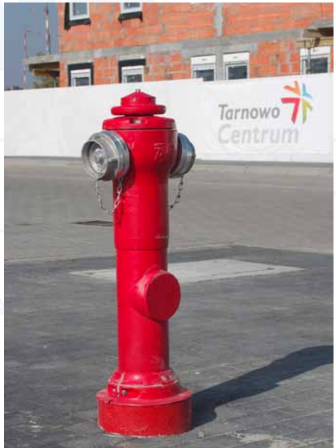
A VEGA hydrant series 78 installed in Tarnowo Podgórze city - 30 km from Pniewy. Sent in by Wojciech Pilc, AVK Components sp. z o.o.
