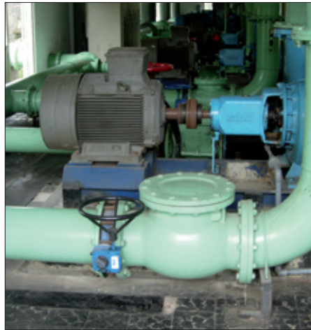
We supplied our wafer type butterfly valves to PDAM Tirtanadi in Medan during year 2003 and today they are still working well in the water treatment plant.
