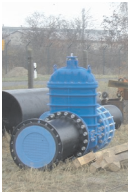
Gate valves pre-assembled for installation.
