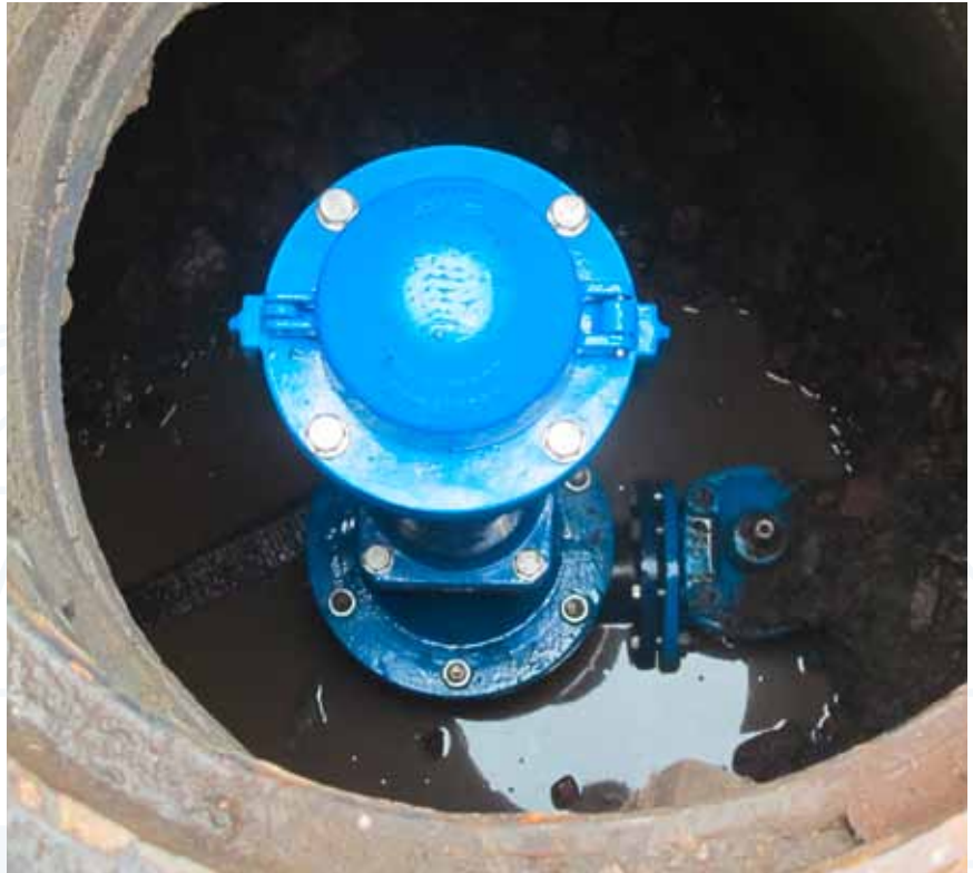
A series 35/72 underground fire hydrant is being installed in Russia. Sent in by Marina Kovaleva, Santeh-Servis
