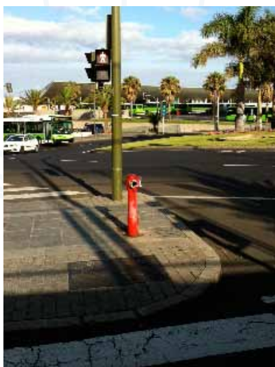
An AVK hydrant in Santa Cruz, Puente General Serrador on Tenerife. Sent in by Jürgen Düllä, AVK Mittelmänn Armaturen GmbH
