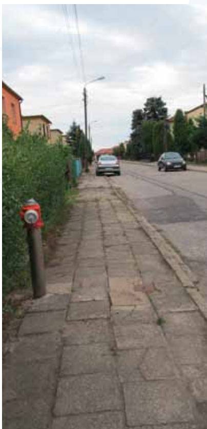
An AVK series 87 hydrant in the city Szamotuly in Poland. Sent in by Inga Wisniewska, AVK ARMADAN Sp. z o. o.
