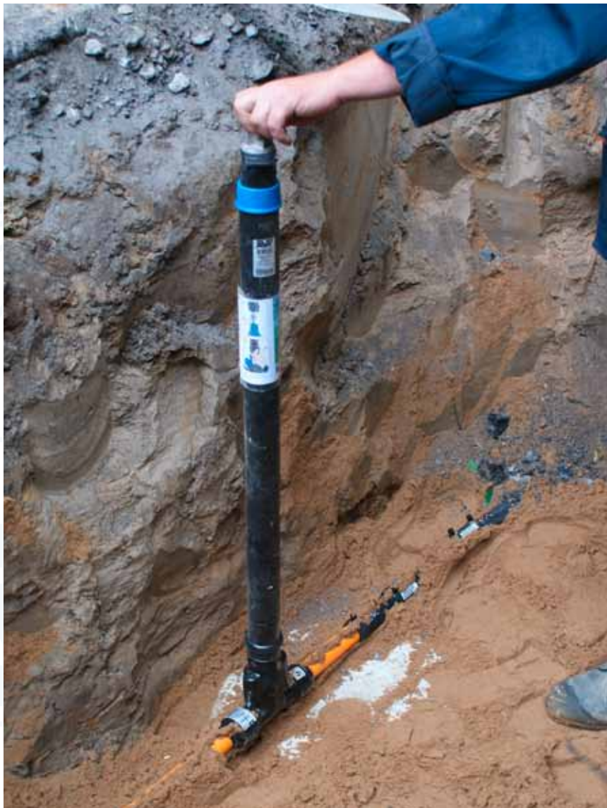
A series 36/90 service connection valves with extension spindle being installed in Russia. Sent in by Marina Kovaleva, Santeh-Servis.
