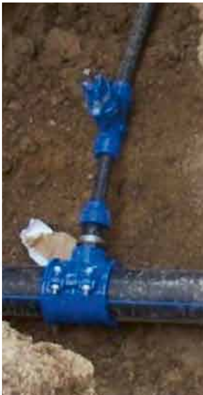
A series 03/30 service connection valve and a series 10 tapping saddle being installed in Russia. Sent in by Marina Kovaleva, Santeh-Servis
