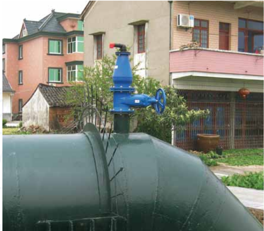
Project: "waste water released to sea after initial treatment", the diameter from DN 1000 to 1400 over 70 km, in Tongxiang City of Zhejiang Province, China. The customer used over 100 pcs. 701/70 sewage air valves. Sent in by Hu Bing, Marketing Director, AVK Valves (Shanghai) Co., Ltd.
