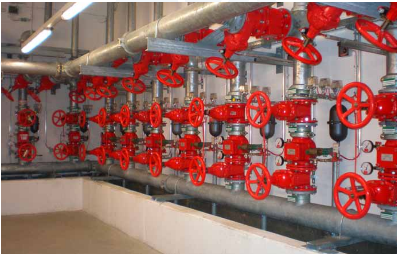
A sprinkler room at Airport München. About 600 valves are built in. Sent in by Eckhard Matz, AVK Mittelmann Armaturen GmbH.
