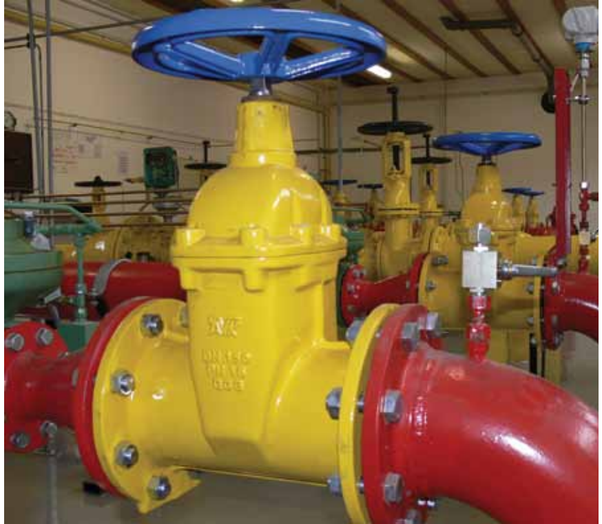
AVK gas valves in a gas works, sent in by Reinhold Rudnik, AVK Mittelmann Armaturen GmbH
