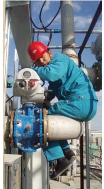
Karamay Petroleum Sewage Plant of Xinjiang Autonomous Region, west of China - sent in by Earnest Hu, AVK Valves (Shanghai) Co., Ltd.
