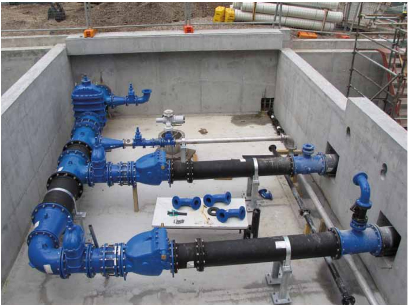
A pit construction at Neutral Bay in the Sydney metropolitan area with the AVK valves being installed.
