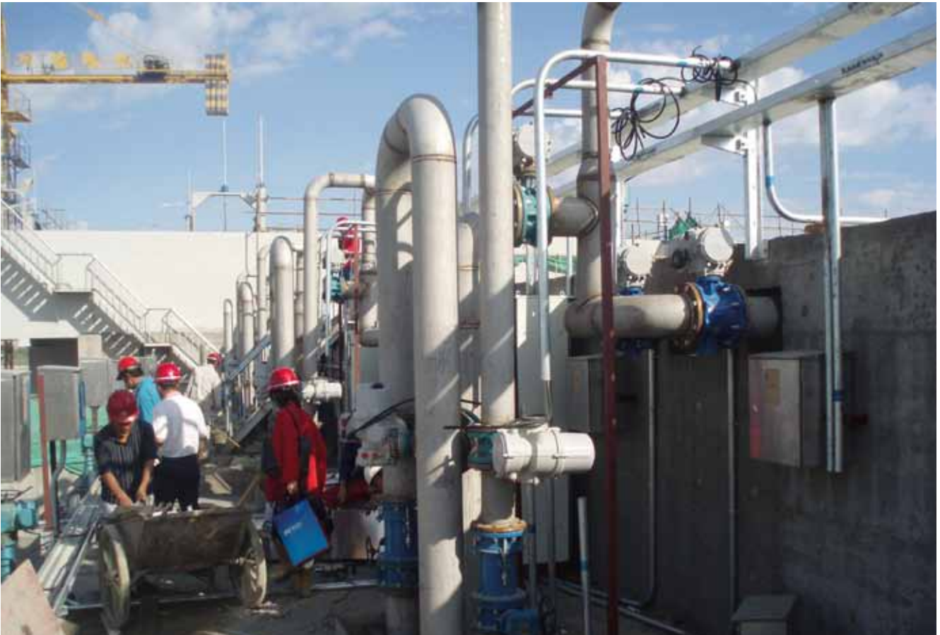
Karamay Petroleum Sewage Plant of Xinjiang Autonomous Region, west of China sent in by Earnest Hu, AVK Valves (Shanghai) Co., Ltd.
