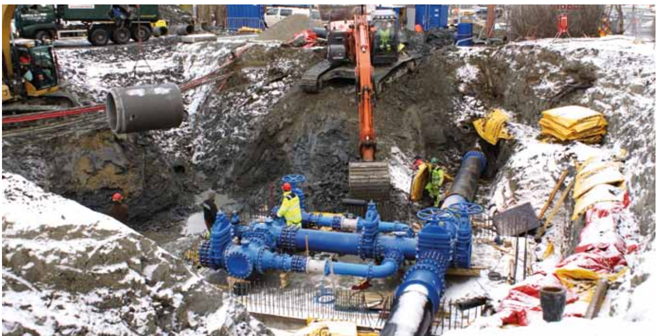
Picture from Trondheim - DN 700 ductile iron pipe main line chamber delivered by AVK Sent in by Svenn Tage Austmo, area manager, AVK Norge AS
